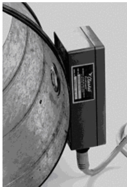
PyroGuard Sensor mounted on pipe
